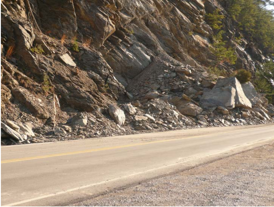
Rocks precariously sit near the road's edge.
