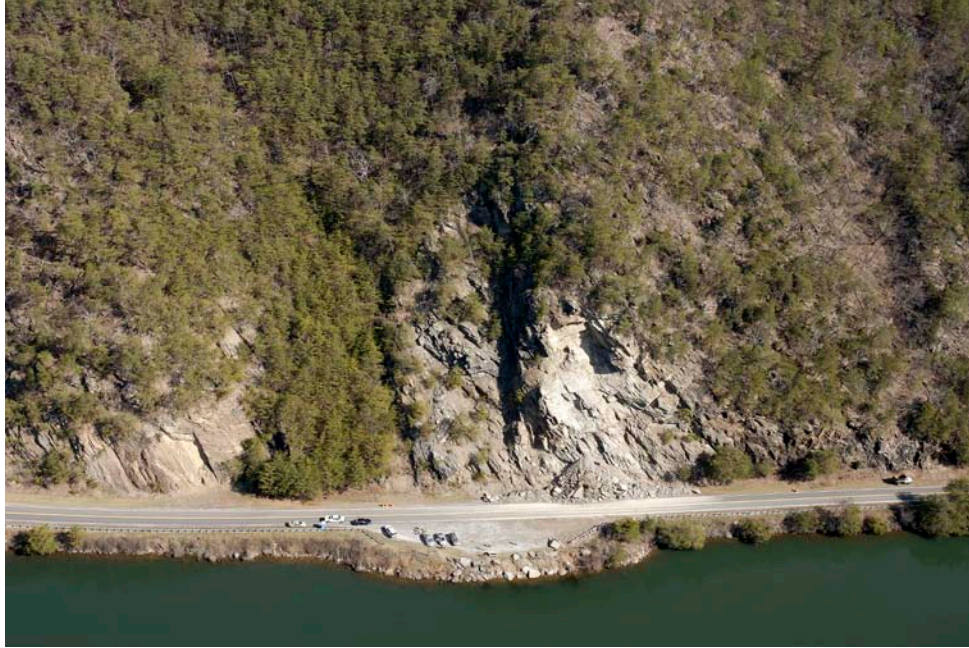
Aerials of rockslide on US-129.
